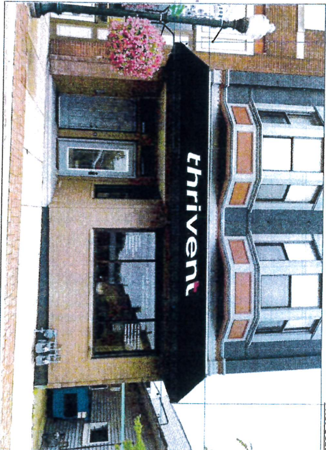
Awning fabric to be replaced
